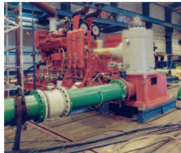
SPP Vertical Turbine pump on test
